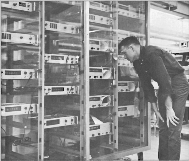
Westbrook gazes at counters held in chamber at 148 degrees F. to detect "temperature-touchy" components.
